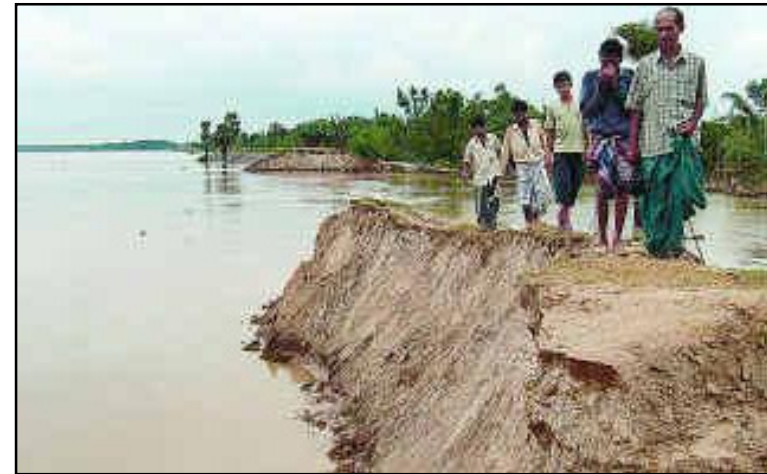
Fig. 7: Local residents on a stretch of the broken embankment
